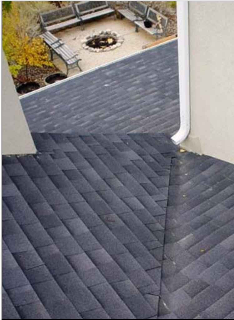
Drainage down this valley will flow against the stucco wall
