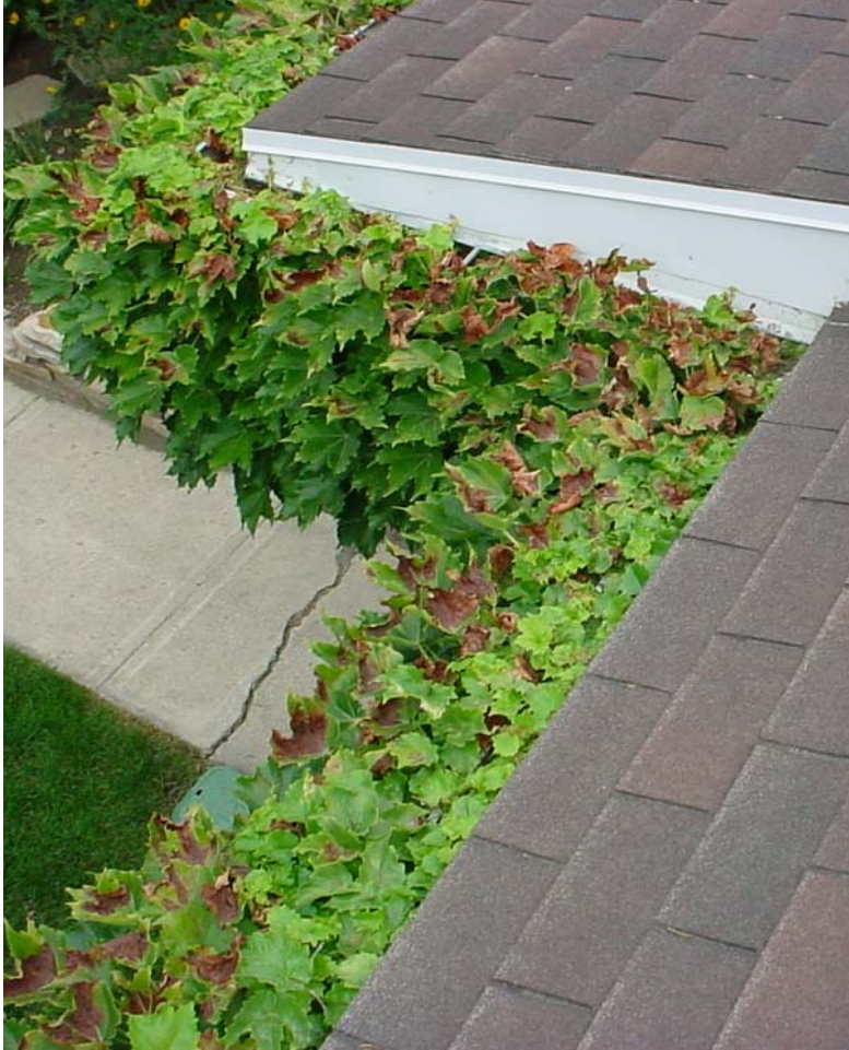
There really are rain gutters on this roof, but they may have some trouble draining
