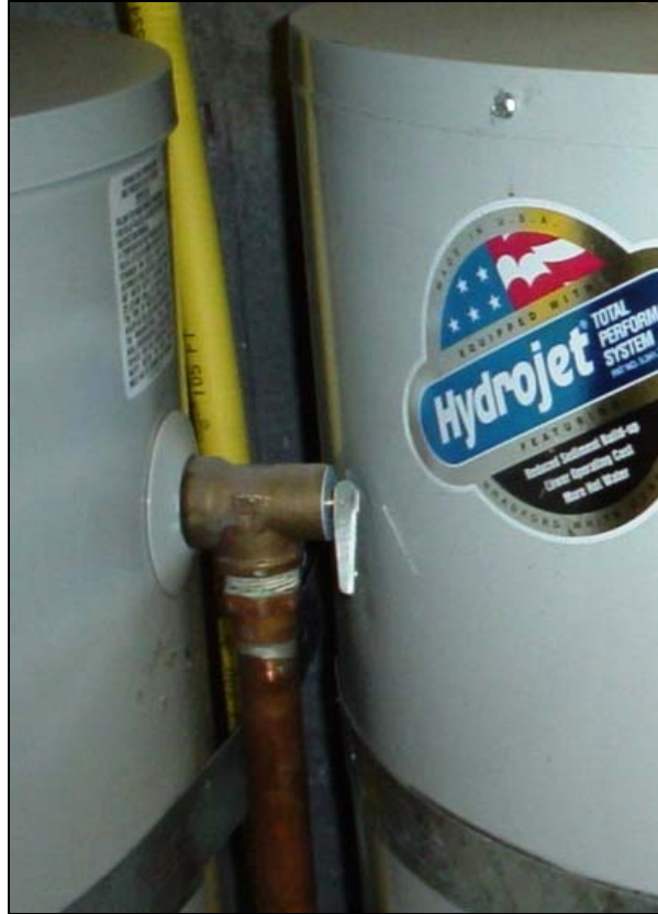
The water heater PRV. This one can't function because it's blocked by the heater next to it
