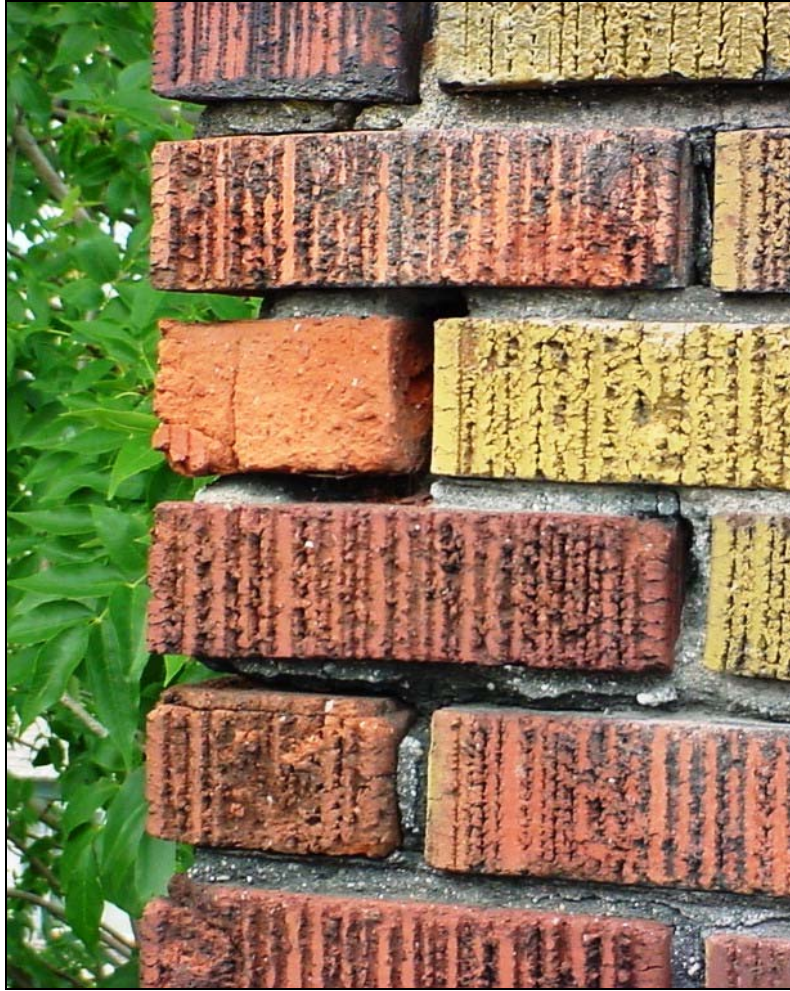
Missing chimney mortar – notice the absence of mortar on the left edges
