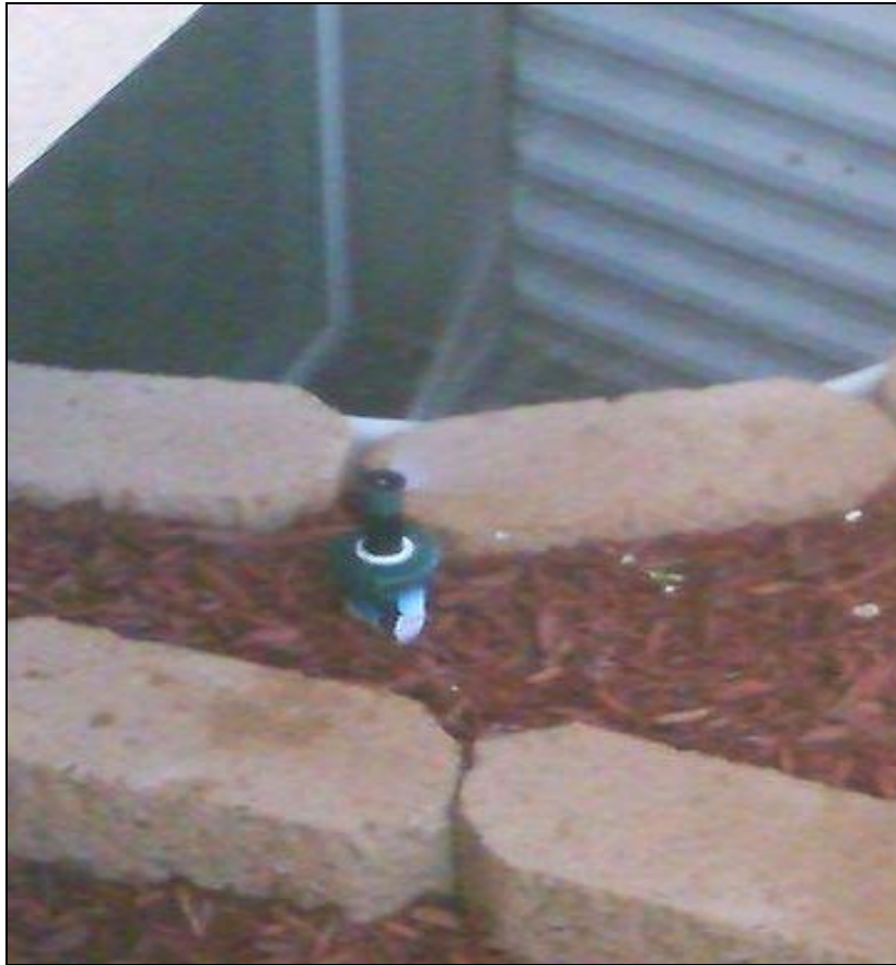
Sprinkler spraying over the window well – this is begging for trouble
