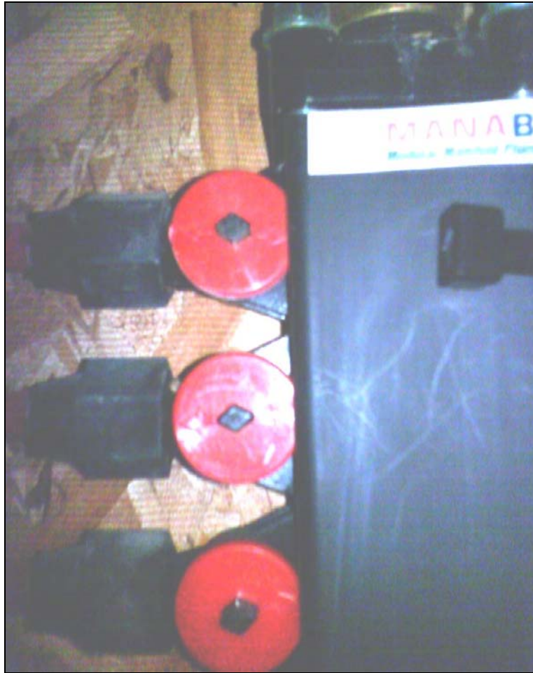
The hot side of the mana-bloc system. Notice the key in the bloc at upper right
