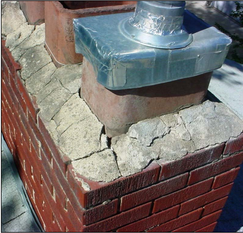
This chimney cap needs to be rebuilt
