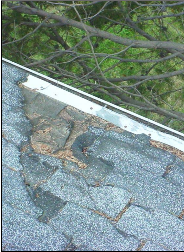
Damaged roof from blowing branches against the shingles
