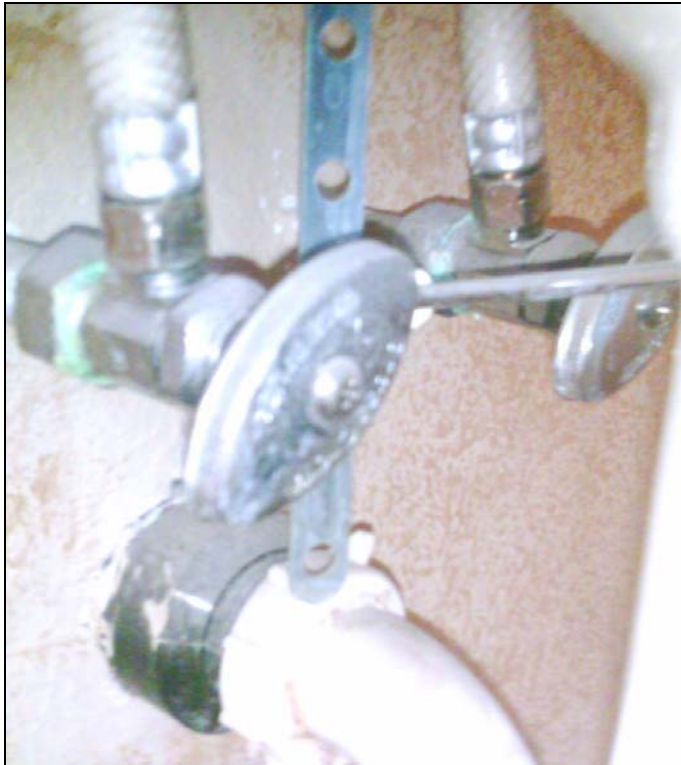
There they are, under the sink. Turn them often.
