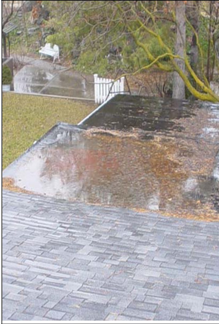
Ponding on a flat roof at center. Notice the reflection of the trees in the ponding water
