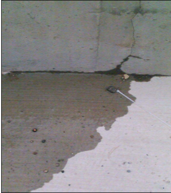
This should leave no doubt about whether water can leak through concrete
