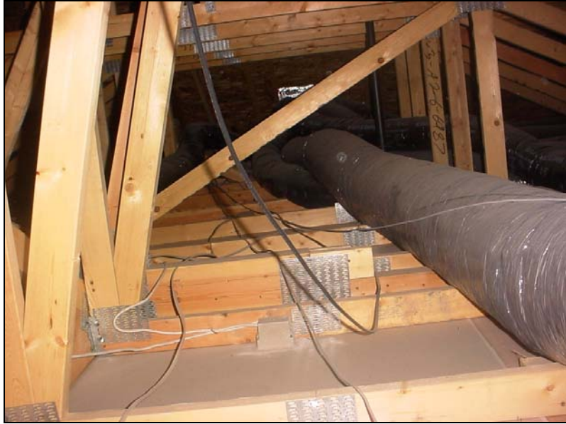
This attic shows the structural components and a heat duct at right. his attic area also lacks any insulation
