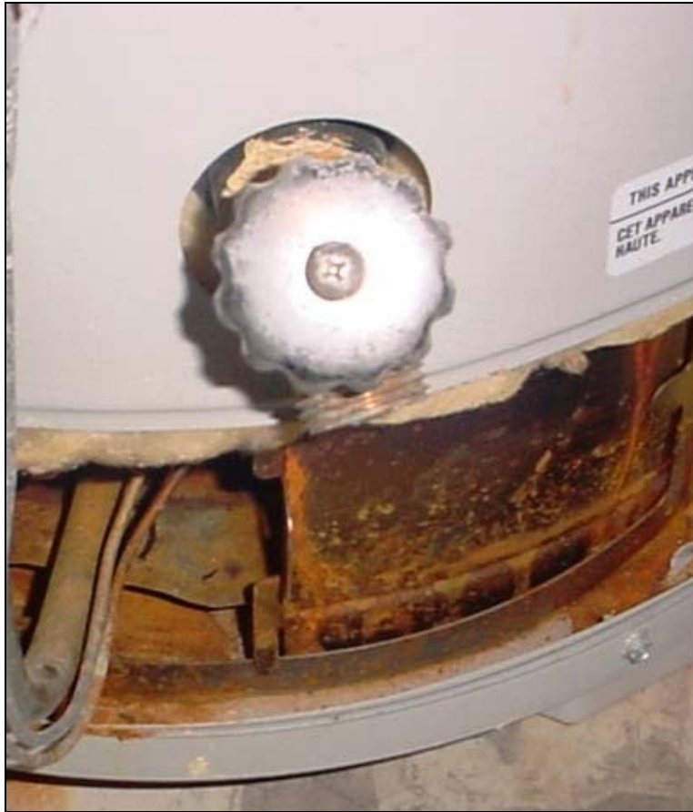
Water heater tank drain valve.
